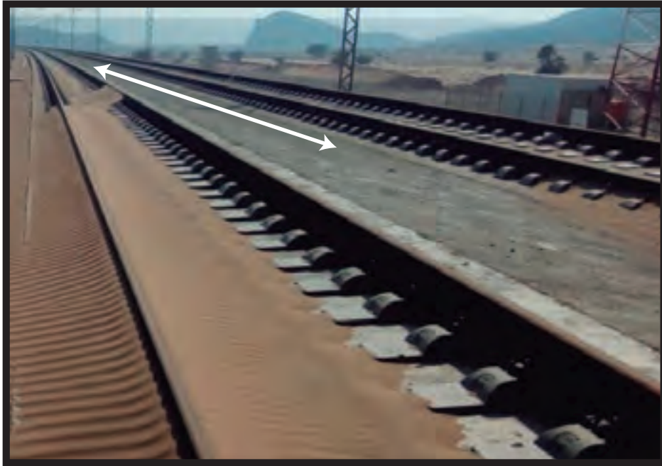
WE CAN OBSERVE THE SAND LACK ON THE RAILWAYS. DUE TO AN AUXILIARY WORK THAT WAS PERFORMED TO PROTECT AN INSTALLATION
