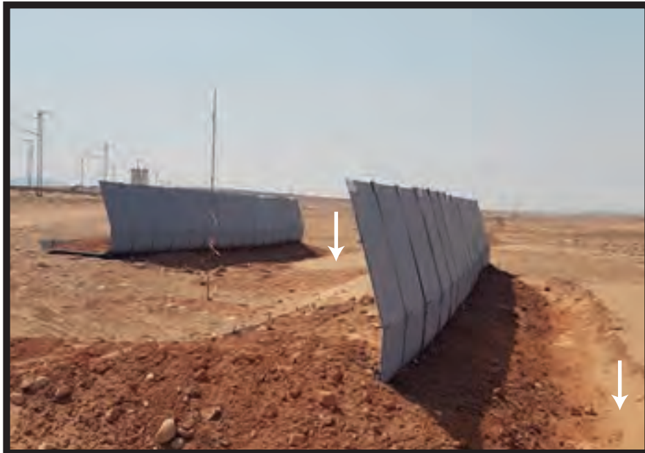
STATUS OF THE SYSTEM MISSING ONE MONTH OF ITS PLACEMENT. IT CAN BE STARTED TO APPRECIATE SAND ACCUMULATION
