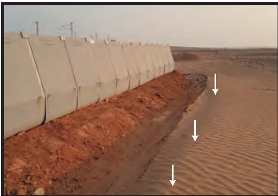
STATE OF THE SYSTEM MISSING THREE MONTHS OF ITS PLACEMENT. ACCUMULATION OF SAND START TO HIGHLIGHT
